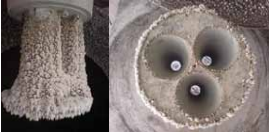
Outer unit is coated with build up from dust
