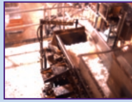
CHUTE PLUG CONTROL
